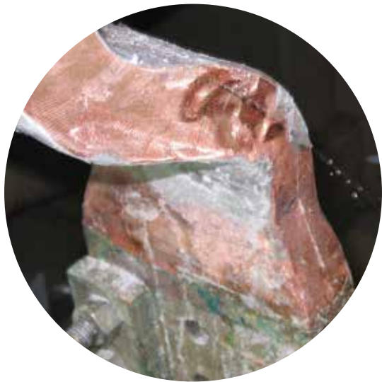
Figure 17. Connection ring braze joint water leak identified during on-site test and inspection
