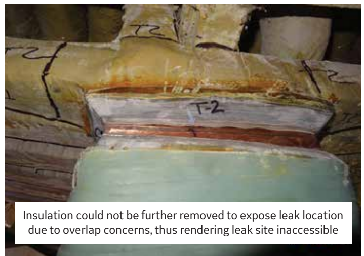
Figure 9. Inaccessible Connection Ring Leak
