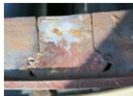
Corrosion typical on carbon steel backing rings
