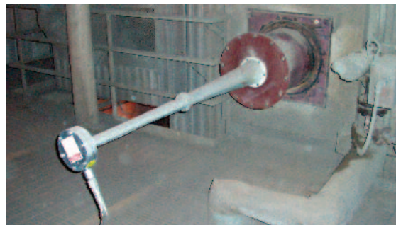
D-75 cleaners were installed in each of the seven access doors throughout the backpass of both 80 MW boilers.
