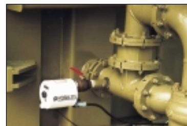
Horizontally on the return pipe from the coolers
