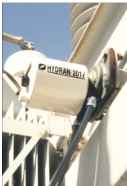
Horizontally on the transformer wall
