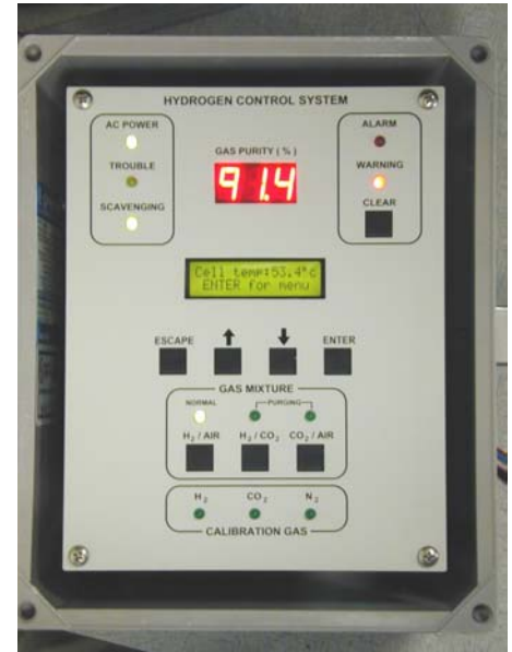
Hydrogen Control Panel
